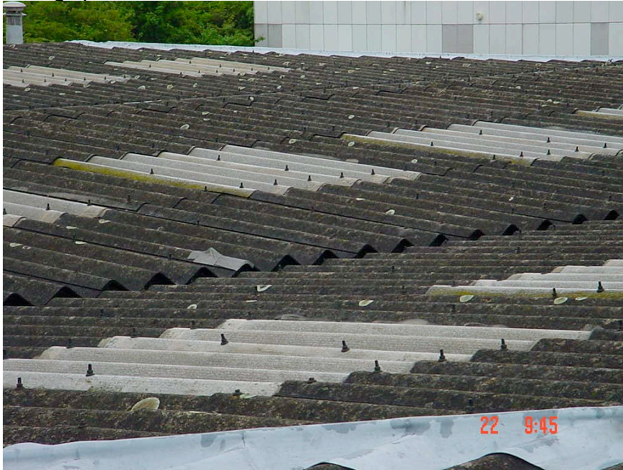
Row 3 Roof light No 2. Flashb and repair to asbestos sheet.
