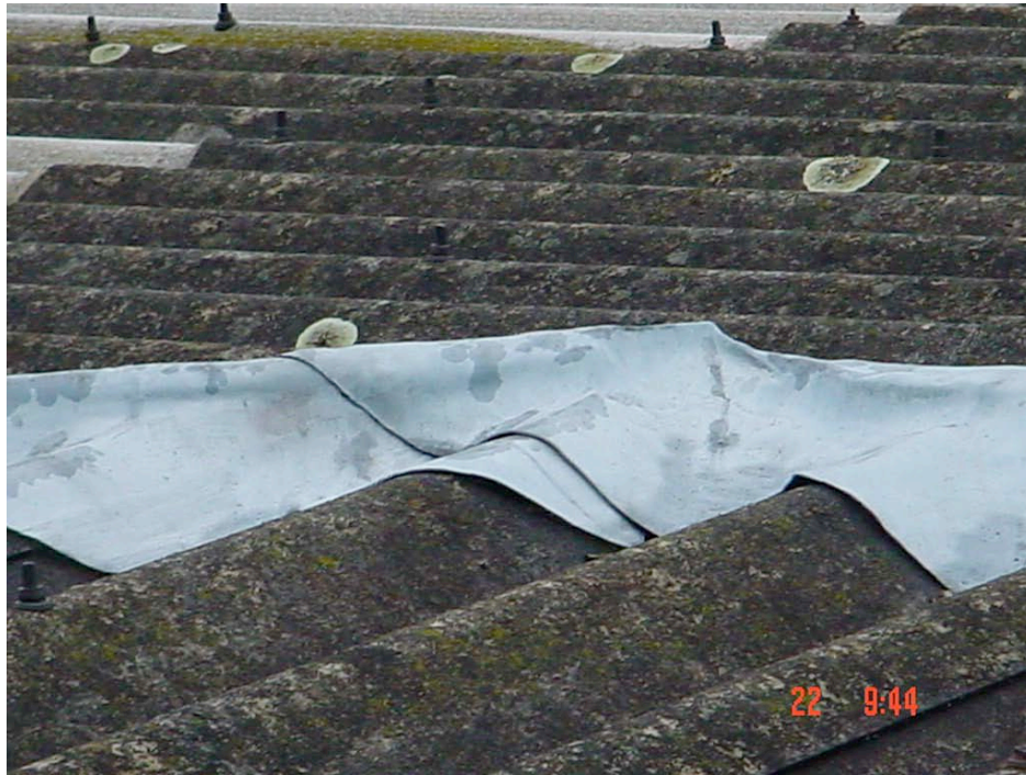
Top of Hip showing poorly dressed lead – could cause splitting.
