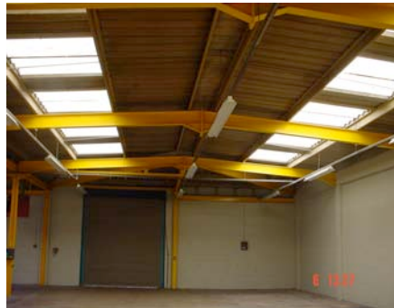
Open Area – Facing Roller shutter door. Note. Possible faulty lights - last two in above rows
