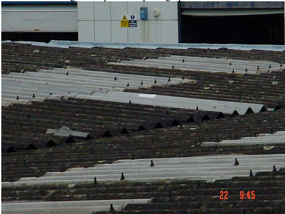
Row No 3. Roof lights 6 and 7. Approximately 5 No replacement asbestos sheets around and under roof lights. Flash band repair by valley gutter.
