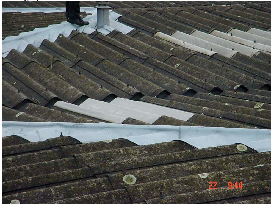
Row No 4. shows replacement asbestos sheet between Roof light No 1 and Front elevation. Note. Chimney to Heater loose [blown off] and vent top to asbestos pipe not fitted [needs new top]
