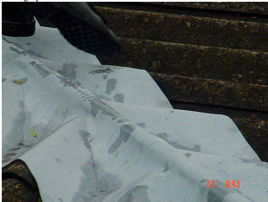
Hip to Row 1 [ over Toilets] Lead Hip has split on top of the ridge. [1/3rds up from bottom corner]
