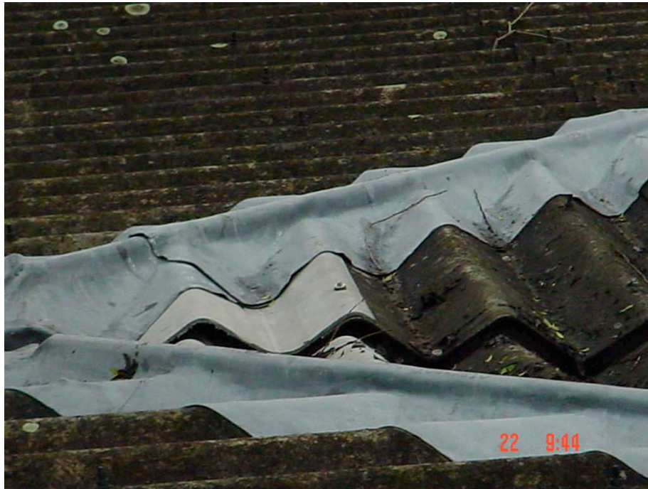
Row 3 Junction of Hips by front Elevation – shows replacement asbestos sheet and redressed hip lead to ridge.
