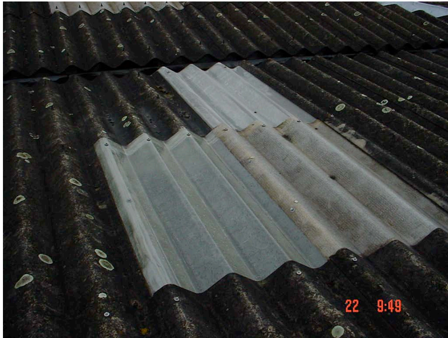
Row No 4. Roof light No 7. New clear Roof light, with adjacent replacement asbestos sheet.
