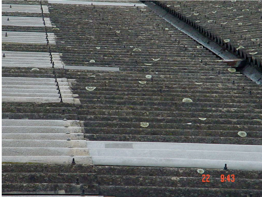
Close up of No 1. Note Possible flash band to replacement asbestos sheet.
