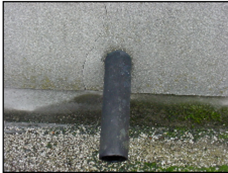
Vertical crack to the wall of the high level roof
