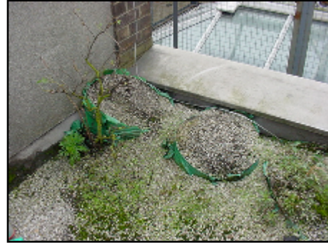
A build up of chipping has occurred in some areas on the roof, these need to be evenly distributed
