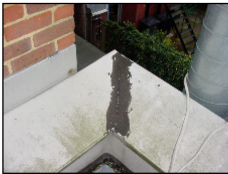
Repairs can be seen to have been previously carried out to the capping
