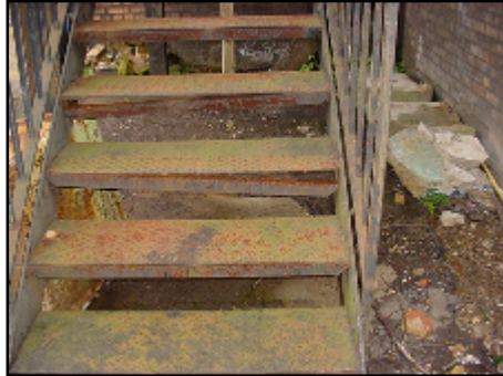
General rusty condition of fire exit
