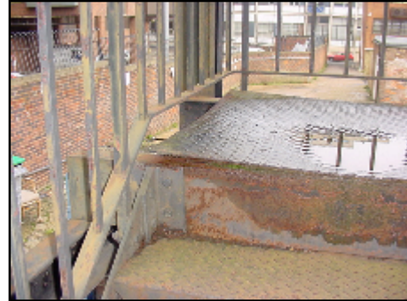
Showing corrosion and metal plate (tread) to have come away from the riser
