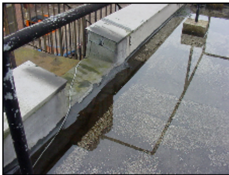
The handrail requires redecoration
