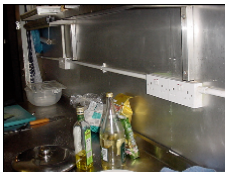
Surface mounted electrics within a cooking area, generally not considered good practice
