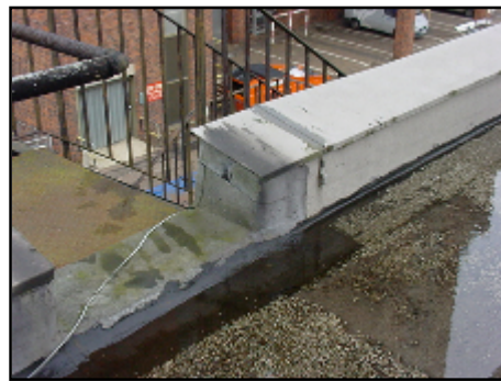
Repairs can also be seen to have been carried out to the roof and the junction of the parapet wall
