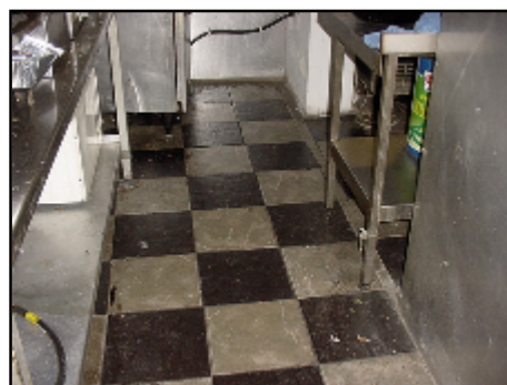
Ingrained dirt and no skirting at perimeter of wall to allow for easy cleaning
