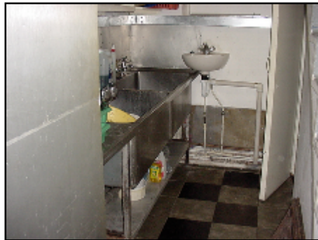
Note ingrained dirt to tiles and pipe work not boxed in
